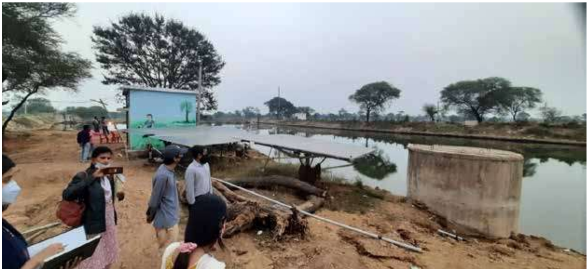
Picture 4 Installation of solar panels near check dam supplying electricity for drip irrigation system
