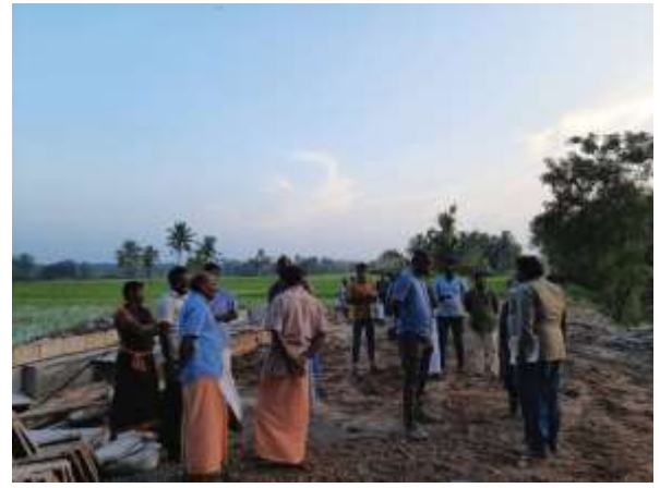
FIGURE 13 In conversation with local farmers and Junior Engineer of the Irrigation Division of Public Works Department, Puducherry. Site of sluice construction for diverting tank water to field channels in Manalipet.
